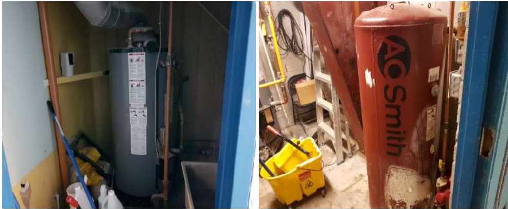
(a) DHW heater
