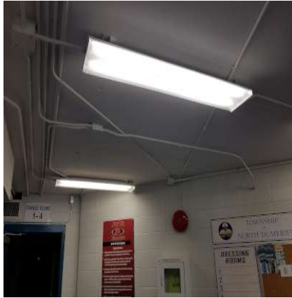
(a) Fluorescent fixtures
