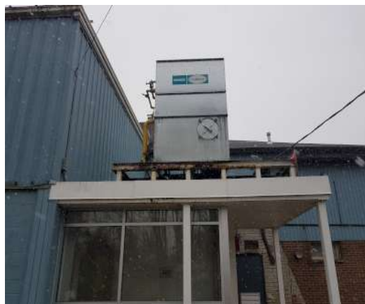
(a) Cooling tower
