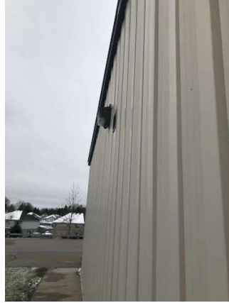
(a) Wallpack Figure 12: Exterior lighting
