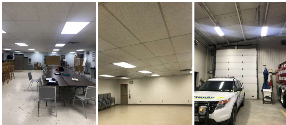
(a) Interior fluorescent fixtures
