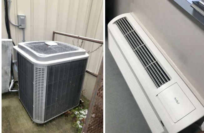
(a) Air conditioning unit (b) PTAC unit Figure 10: Space cooling system
