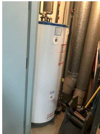
(a) DHW heater Figure 11: Domestic hot water system
