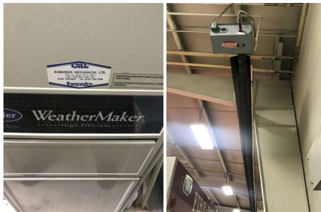
(a) Furnace (b) Radiant tube heater
