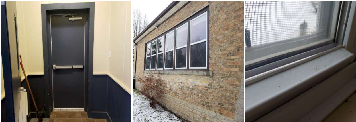
(a) Exterior door
