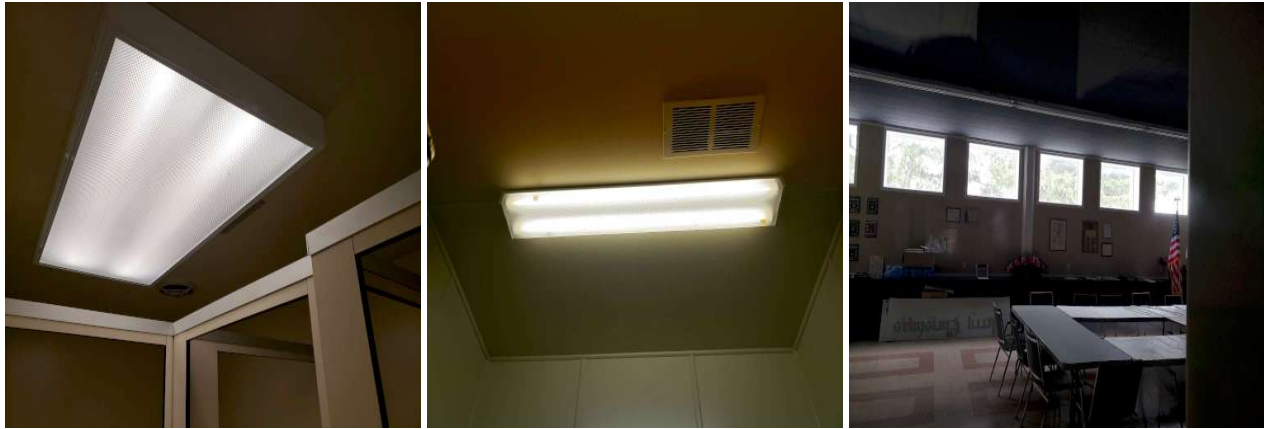
(a) Typical fluorescent fixtures
