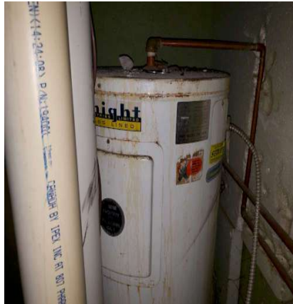
(a) DHW heater
