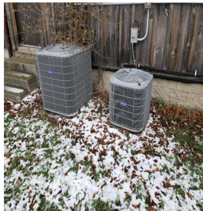
(a) Air conditioning units
