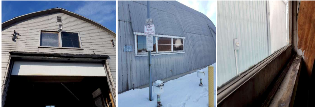
(a) Exterior door
