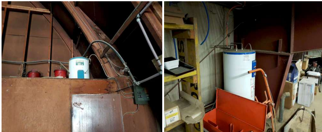
(a) DHW heater
