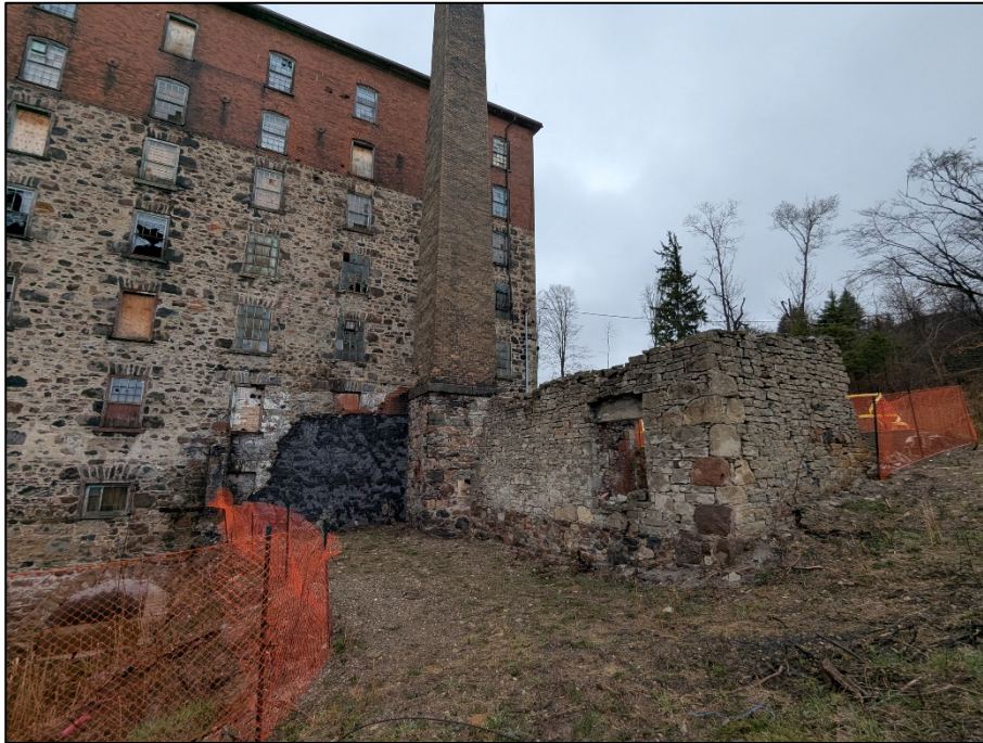
Photograph 4: Ruins and Chimney
