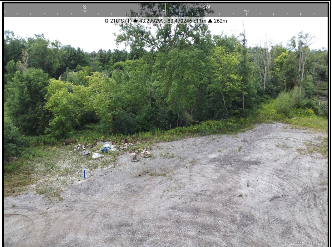
Photo 12: Aug 26, 2025 A view of the southwest portion of the site from the upper level of the mill, looking southwest.
